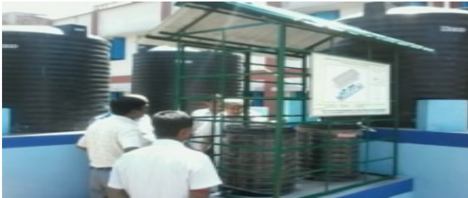
RAIN WATER HARVESTING PLANT
