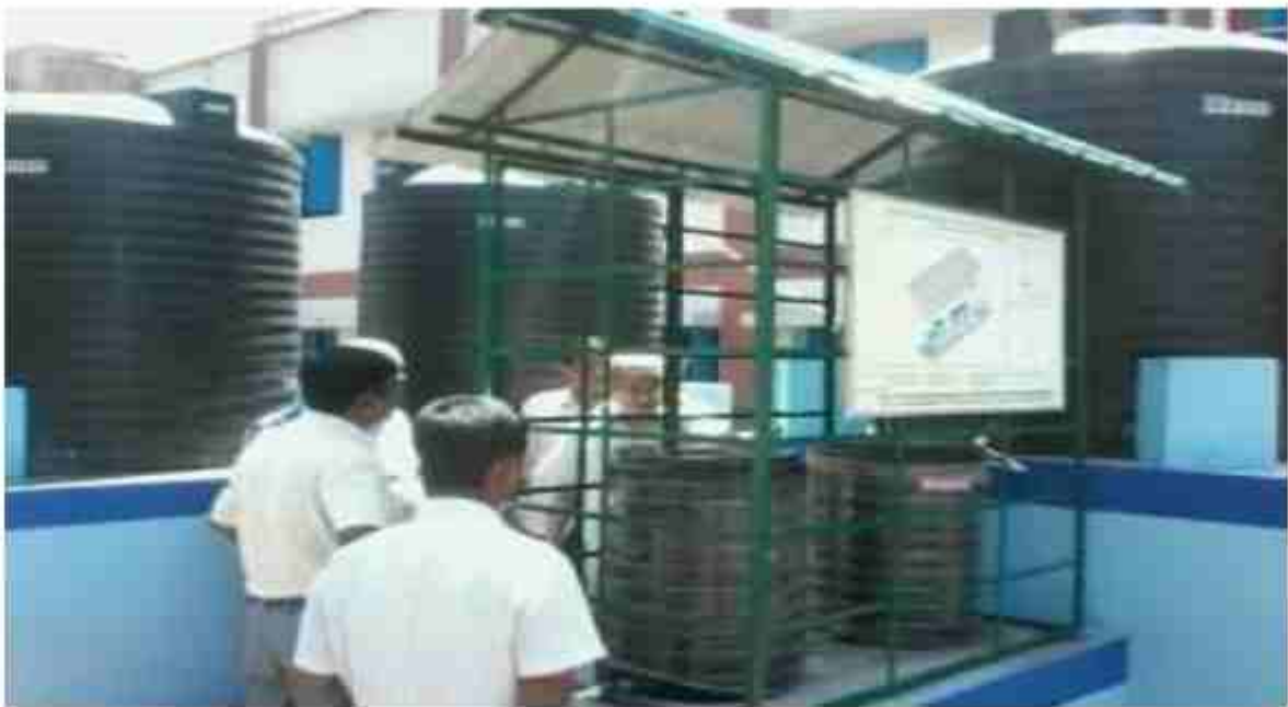
RAIN WATER HARVESTING PLANT, 2016.
